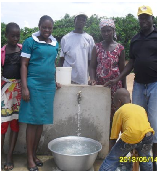
Outside Water Point
